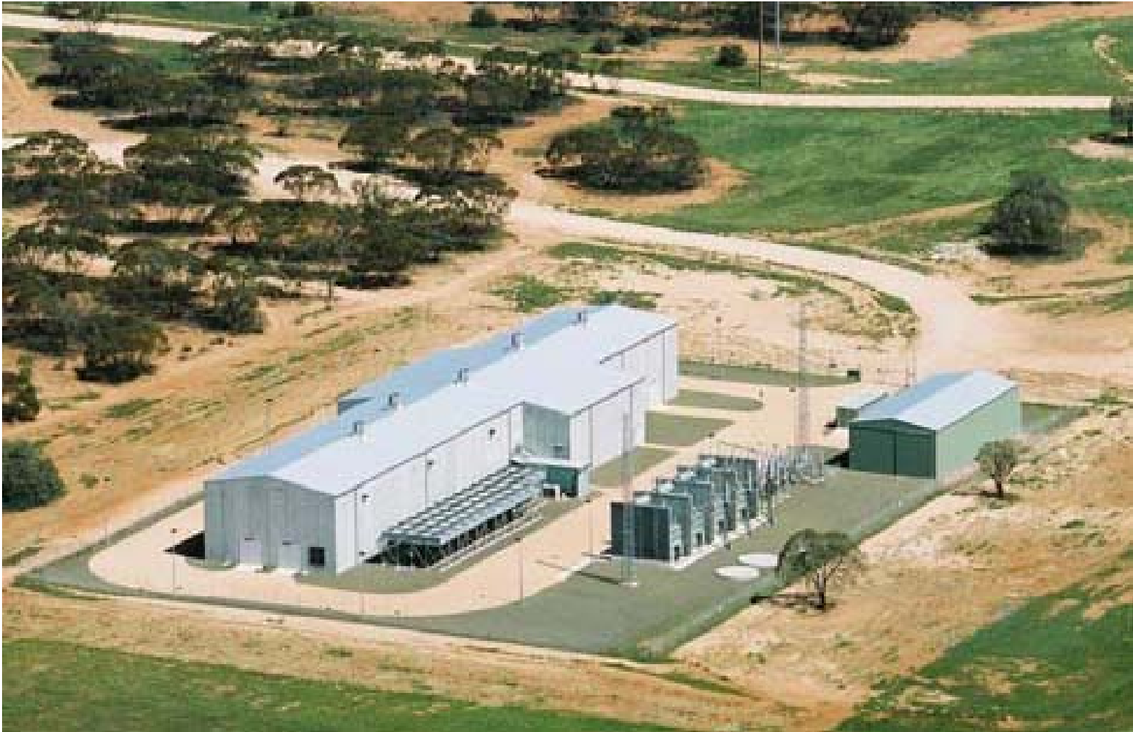
Berri Australia Converter Station ABB Cigre 2010
