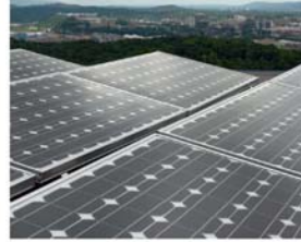
Ruby Falls 16kW Solar PV System in Chattanooga
