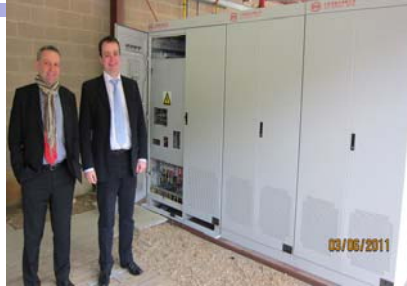
50 kW / 46 kWh BYD system
