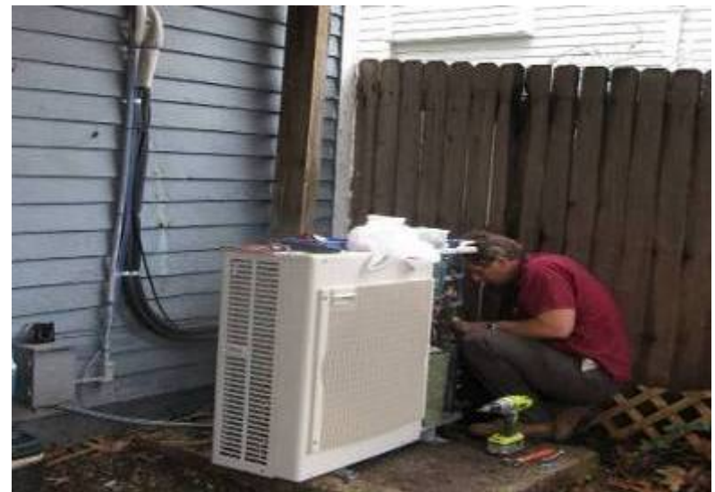
Installation in Chattanooga, TN (TVA)
