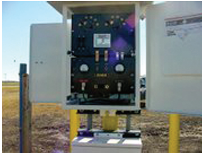
Figure 3-7 Cathodic Protection Rectifier Connected to a Pipeline
