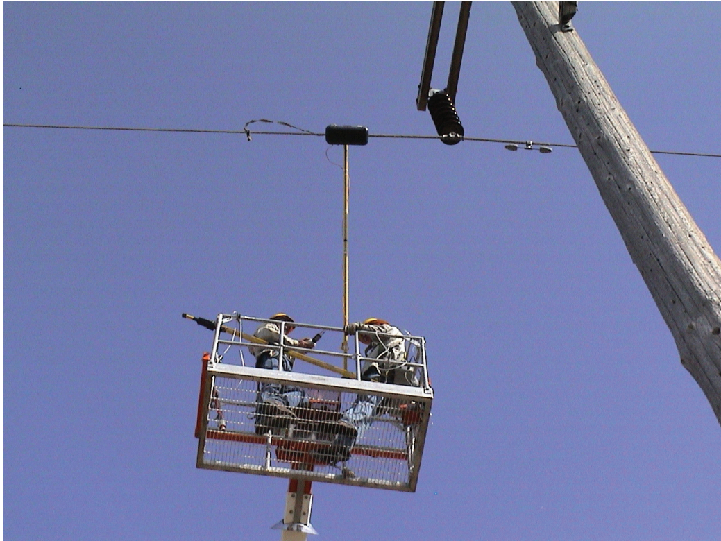
Figure 3-6 Energized Implementation of EPRI EMAT Device to Inspect for Broken Strands Internal to the Conductor Shoe
