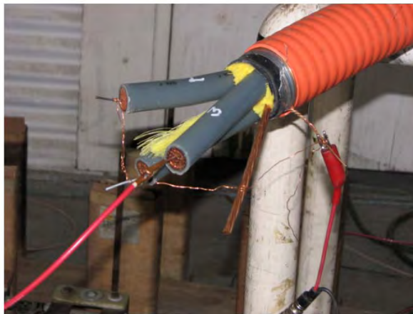
Connection of cable sample during DF measurement at 60 Hz.
