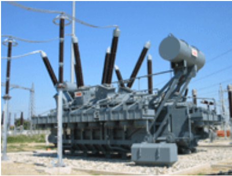
Phase shifter transformer
