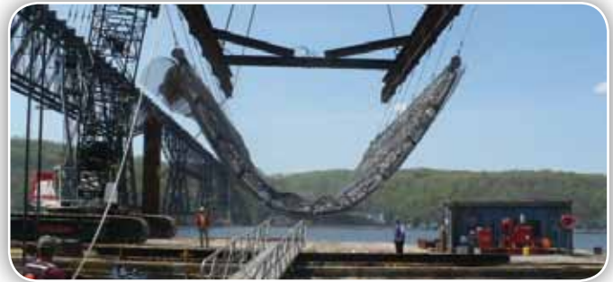
Sorbent-filled marine mattresses are lowered into the Hudson River to test their effectiveness in cleaning up coal tar residues.
