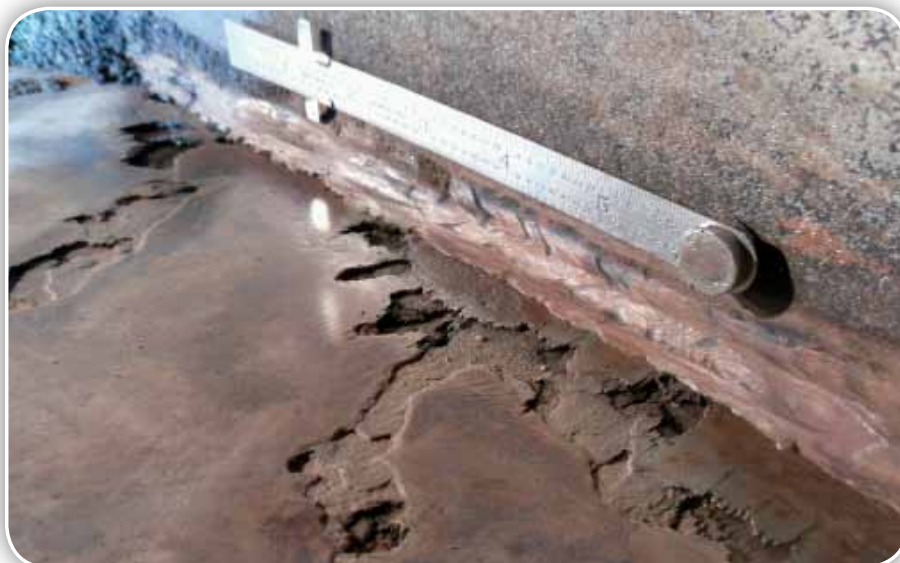
Corrosion damage at a wall and floor joint
