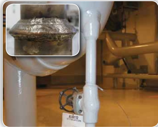
Nuclear power plants have thousands of socket welds that are susceptible to fatigue failures.
