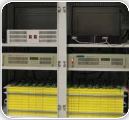
EPRI tested this 6-kW/20-kWh lithium-ion battery system at its Knoxville laboratory and is planning to evaluate a 25-kW/50-kWh scale-up by the end of the year. (Photo courtesy Greensmith Energy Management Systems)
