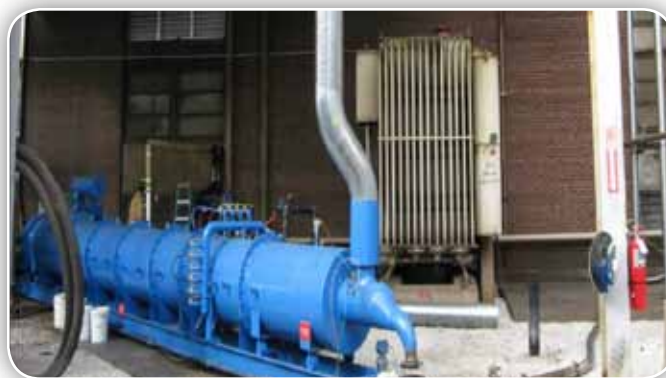
Full-scale prototype sorbent activation unit, installed at a power plant.
