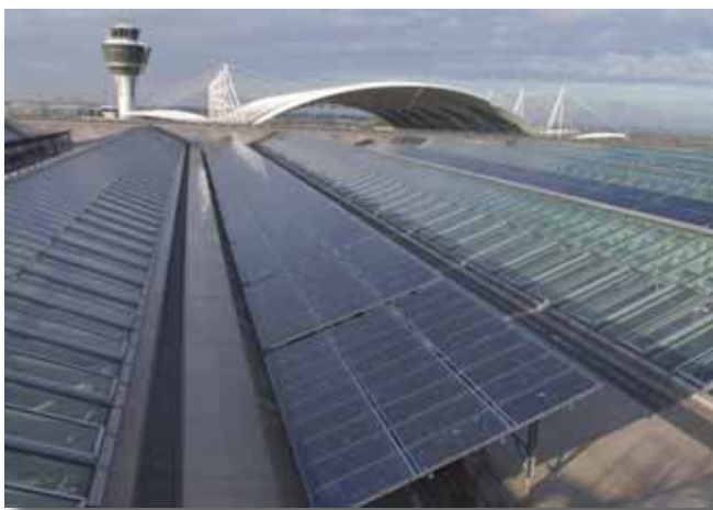
Silicon photovoltaic systems engineered for low maintenance and long-term environmental exposure are being used increasingly on commercial buildings worldwide. This 457-kW array was installed on the roof of the Lufthansa terminal at Munich Airport in 2002. (photo: BP p.l.c.)
