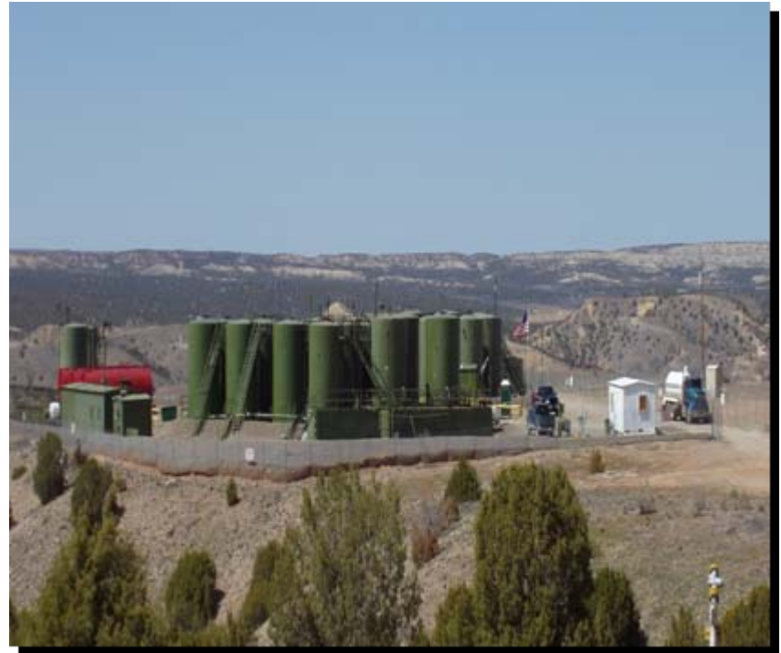
McGrath Salt Water Disposal Facility (SWDF)
